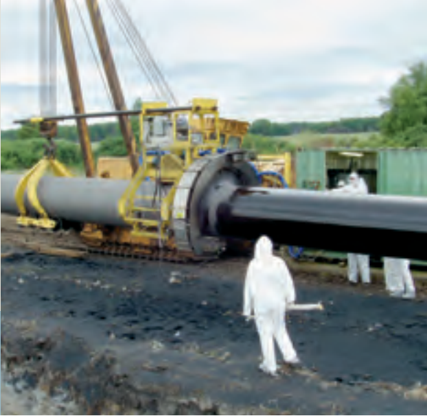
Pipeline rehabilitation applying PROTEGOL®UR Coating 32-55 over the ditch at a location in Czeljabsinsk region, Southeast Ural, using automatic spray unit with three oscillating guns as the method of application (Courtesy of Incal Pipeline Inc.)
