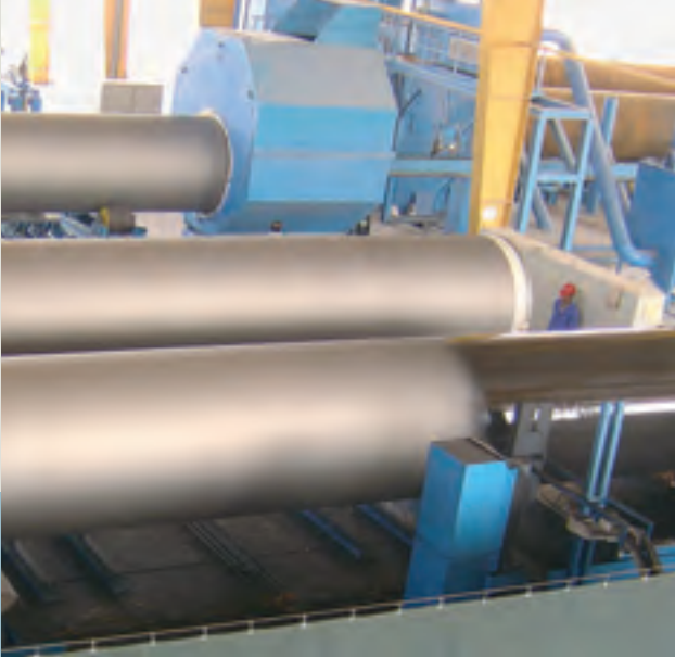
Online coating facility for coating of pipes with different pipe diameter: Blasting unit/buffer zone/pipe coating section
