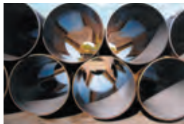
Online application for internal lining of 56" pipes with PROTEGOL®EP Coating 130 HT, in a coating thickness of 600 µm
