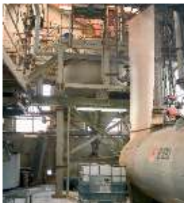
Spent flux recycling plant
